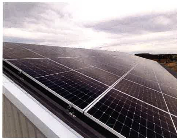
WYOIT LLC received a REAP grant to purchase and install photovoltaic solar panels that will generate 41,360 kWh (kilowatt-hours) annually, enough energy to power three homes.
