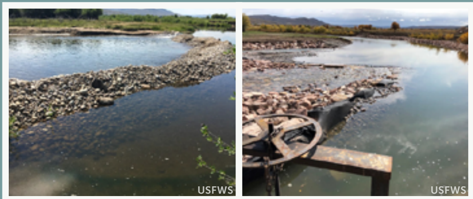
Before (left) and after (right) a diversion structure improvement. This work likely reduces entrainment and improves passage both directions past the diversion. Nick Scribner, WGFD
